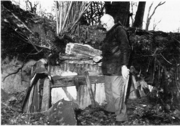
Wiston OB: former Royal Engineer, Laurie Tooth, inspecting the remains of his wartime construction
